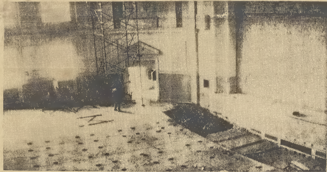
REMODELING MEMORIAL HALL —The entire auditorium of Memorial Hall is currently undergoing extensive remodeling while new seats are being installed. Built 25 years ago, Memorial Hall has been noted for its uncomfortable wooden benches since that time. News Leader Photo
