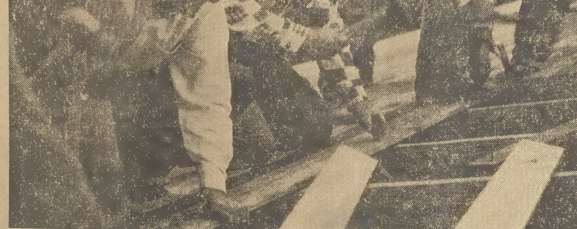
FULL SPEED AHEAD—Construction of Chapel Hill's new Amity Methodist Church is pushing full speed ahead with a volunteer labor force. Shown working on the church roof are Burnice Sparrow, Donald Sparrow, Howard Stewart, Dallas Durham, Herman Greene and Floyd Brockwell.
