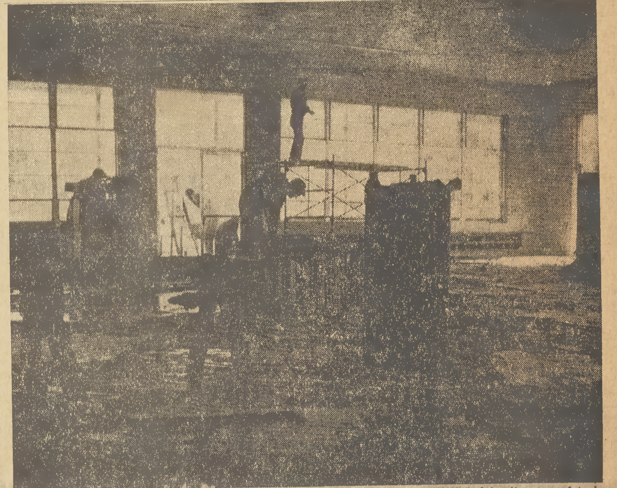
WORK PROGRESS—Shown above is the dining section of Chapel Hill High School's new cafeteria, which is scheduled to be completed within two weeks. When the picture was taken, workmen were watering and cleaning the tile floor. The kitchen of the cafeteria is to the right of the picture.
