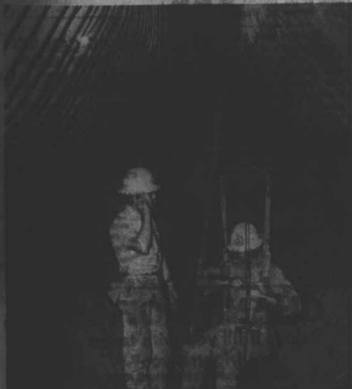
THE LONG RIDE—These two mechanics stand in the ash hopper of CP&L's L. V. Sutton steam-electric plant at Wilmington. Joseph Fips (right) straps himself into harness for a ride to the top of the 150-foot boiler to sandblast boiler tubing. L. B. Smith gives telephone directions to the winch operator. When the plant is in operation, this area is filled with water to carry off fly ash from the combustion chamber above the furnace throat (opening at top).
