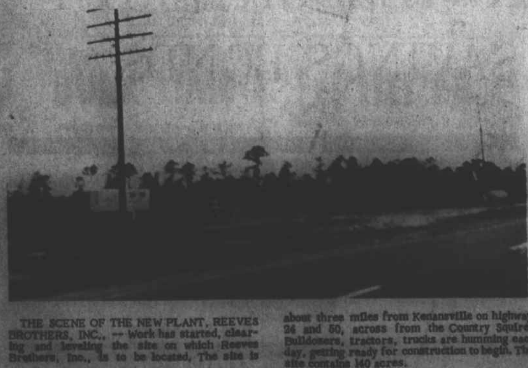
THE SCENE OF THE NEW PLANT, REEVES BROTHERS, INC. -- Work has started, clearing and leveling the site on which Reeves Brothers, Inc., is to be located. The site is about three miles from Kenansville on highway 24 and 50, across from the Country Square. Bulldozers, tractors, trucks are humming each day, getting ready for construction to begin. The site contains 140 acres.
