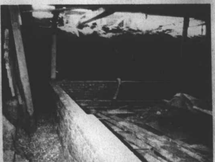
Work in the basement at Liberty Hall moves slowly. The top picture shows the opening into the basement which caved in when the water level was found to be only five or six feet below the ground surface. In the middle picture, the bulldozer is shown moving away the muck and mire from underneath the house. In the bottom picture, one can see the walls of the basement rising, and beside the wall is the gravel and tiling which will drain all water off and keep the basement dry for a home for the heating and air-conditioning system of the house.
