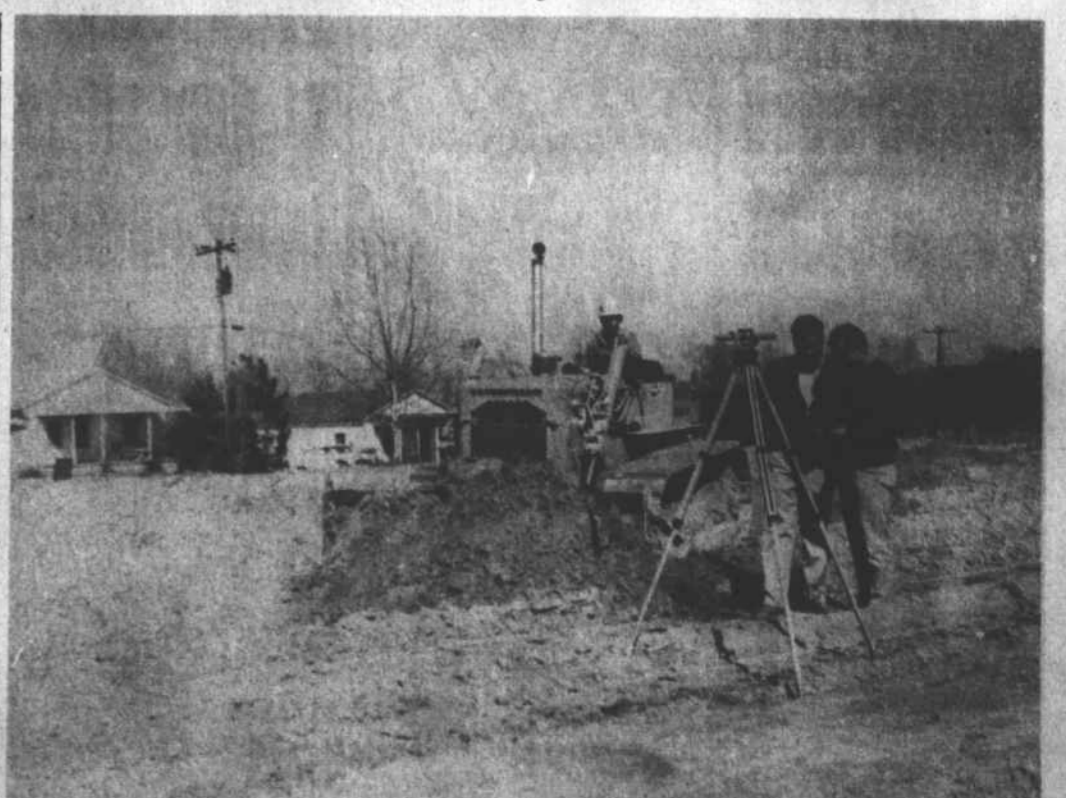
Prior to laying the foundation for the Whaley Rest Home in Kenansville, D. J. Fussell Co., building contractors of Rose Hill, level the ground for the modern, all electric structure
