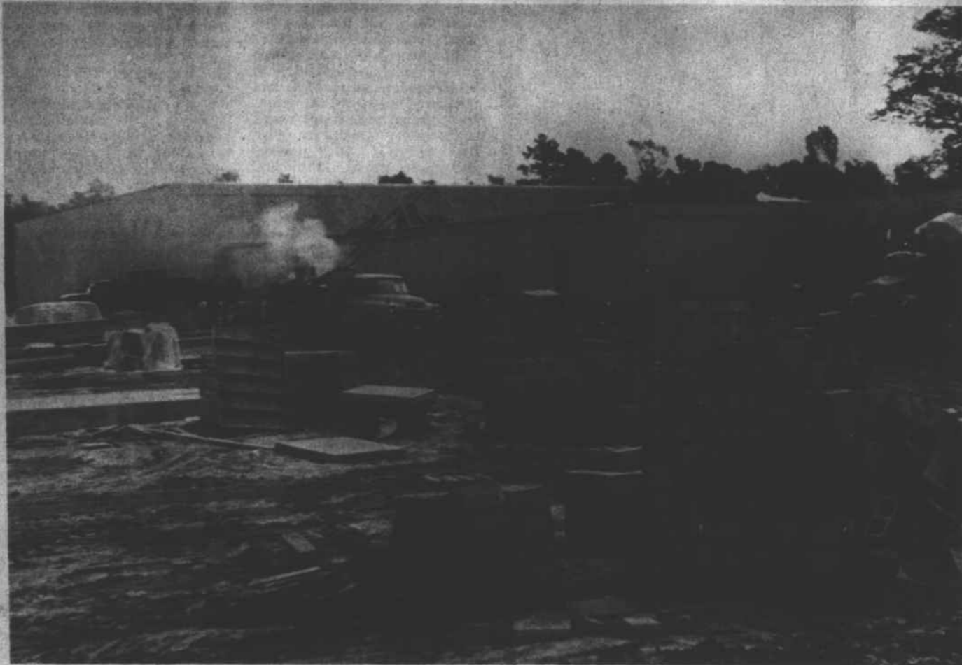
The Turkey Processing Plant near Wallace is approaching final stages of construction with tentative plans for beginning processing operations October 1st. The 60,000 square foot structure will bring to the area the most modern facilities available for processing and freezing turkeys. (Photo by Ruth B. Wells).
