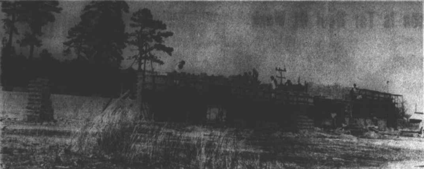
Construction progresses at a rapid rate on the building in Rose Hill which will be the home of new industry. A corporation has been formed by civic minded Rose Hill Citizens to provide this facility which will bring badly needed employment to many people in the area.
