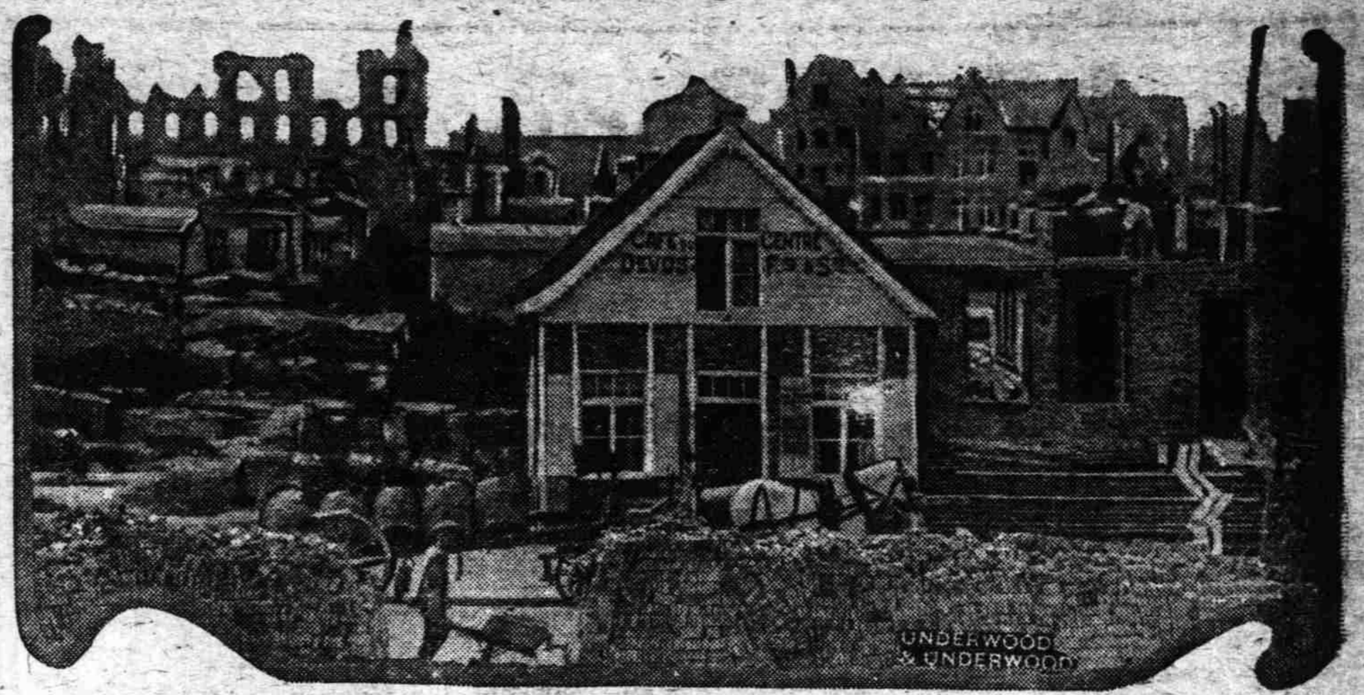
Feverish activity today features the reconstruction of the battle-wrecked parts of Flanders. This photograph shows the builders working among the ruins of Ypres, and was taken by an American Red Cross official, who was accompanying the American Legion delegation on its tour of France and Belgium.
