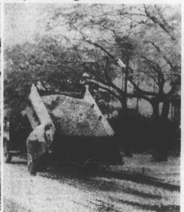
The street has been surfaced with macadam and hot asphalt. It is the first time the street has been paved. The street, which is next to the high school athletic field, will serve as a test street. It will enable town officials to determine the cost of paving other streets in the town.
