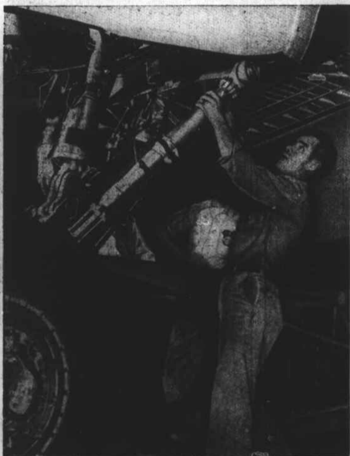
5. Workers guide main landing gear into position. Main gear units fit into inboard engine nacelles; forward leg retracts into fuselage.
