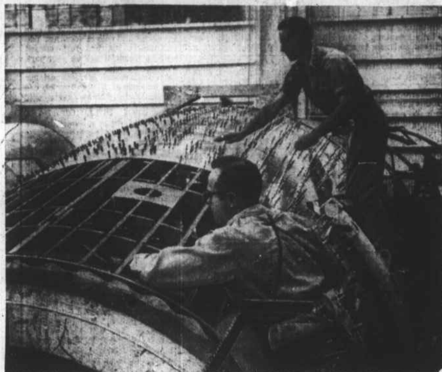
2. Workers affix metallic snap-on fasteners to hold outer aluminum alloy skin position for riveting positions. Fasteners are then replaced by finishing rivets.
