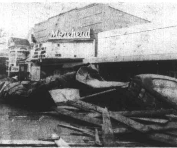
The roof of Freeman Brothers store, in the 700 block of Arendell Street, Morehead City, crashed to the street about noon Friday. Fortunately no one was injured when the heavy mass fell down. Those who heard it said it "made an awful roar." The debris mangled the sign on the theatre and smashed the plate glass window in Belk's.
