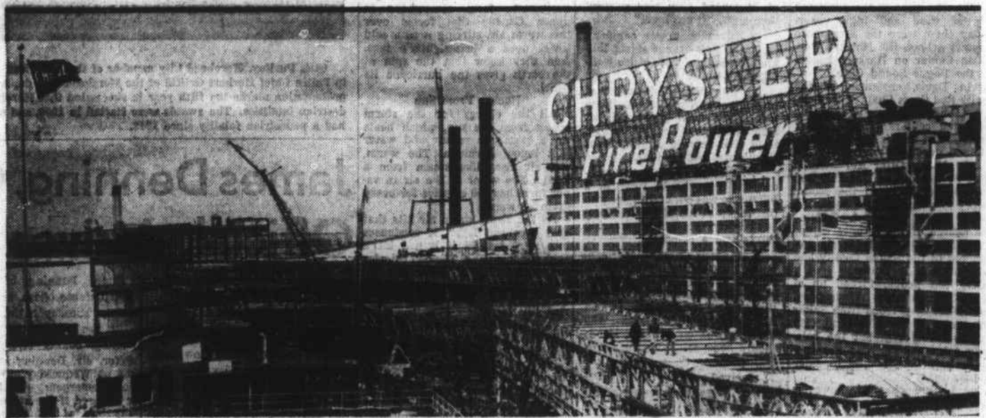
UP GOES CHRYSLER'S PRODUCTION MORE THAN 40% Here you see construction work proceeding on the new Chrysler production facilities which will add 667,000 square feet of floor space . . . including a 1 1/2-mile long continuous conveyor system, longest in the industry.
