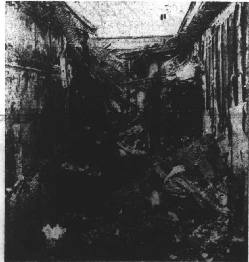
Charred wood and ashes and a wet dismal odor were all that greeted a visitor to the storage area at the rear of the store. (See other pictures page 8 this section).
