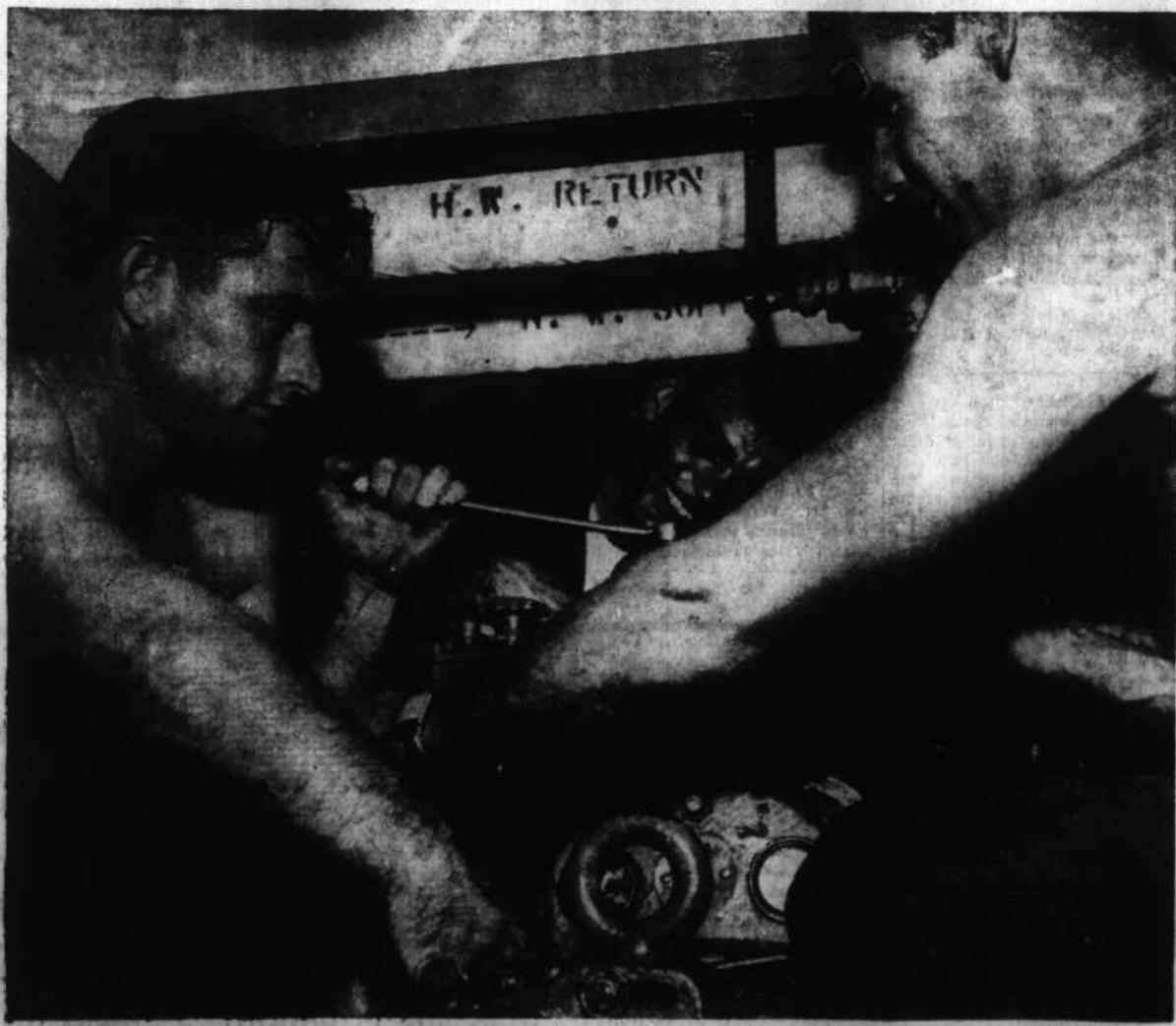
Putting a new diesel injector in one of the two generators on an LCU are, left to right, Sgt. James E. Leary, Morehead City, M/Sgt. George W. Terrell, Havelock, and Sgt. Frank E. Springle, Beaufort.
