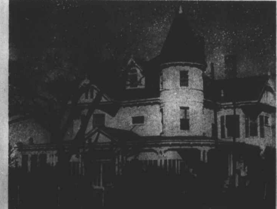
The Charles S. Wallace house as it appeared before workmen started to tear it down several weeks ago. The house is located on the northwest corner of 8th and Arendell Streets.
