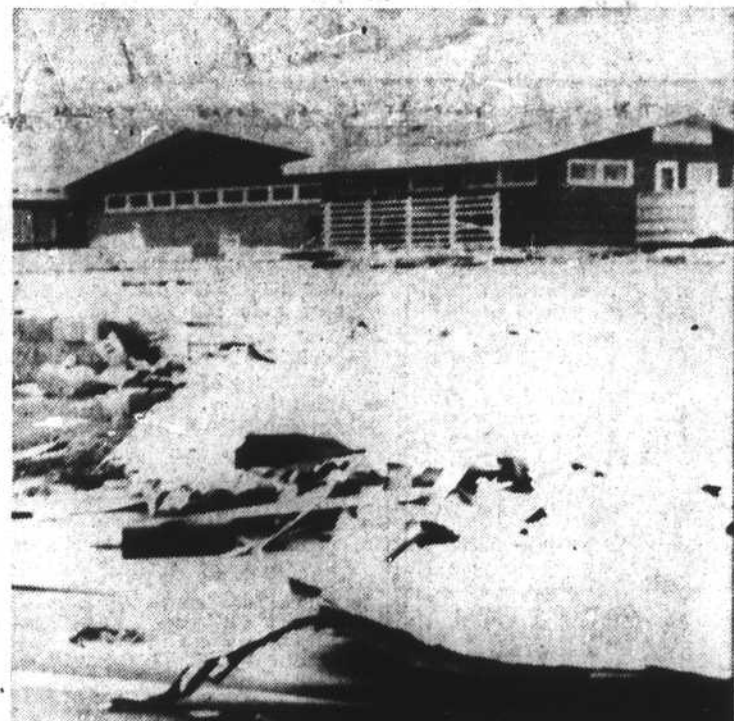
A roof from part of the Coral Bay club lies at the west entrance to the luxurious Bogue Banks recreation spot. Plate glass windows on the oceanfront of the club were blown out. Damage to the club alone will run into tens of thousands.
