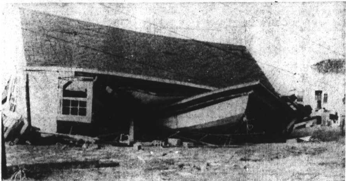
Destruction on the Beaufort-Morehead City causeway alone will total more than a hundred thousand dollars. This house and garage collapsed on top of a boat.
