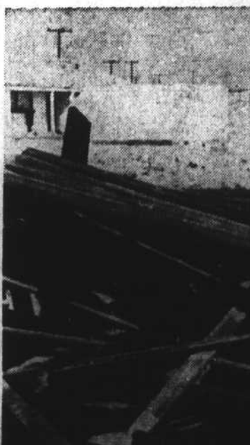
Fall housecleaning jobs like this one face lots of people since Donna passed through. It's clean up and rebuild, a job that will take several months. This is part of the boardwalk at Fort Macon state park.
