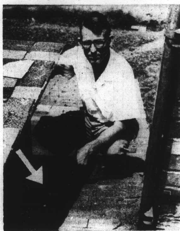
Mike McGowan, Broad Creek, perched on the roof of his house, shows where lightning put a hole through the roof (arrow). The lightning caused several hundred dollars damage to the McGowan home the night of Monday, July 3.
