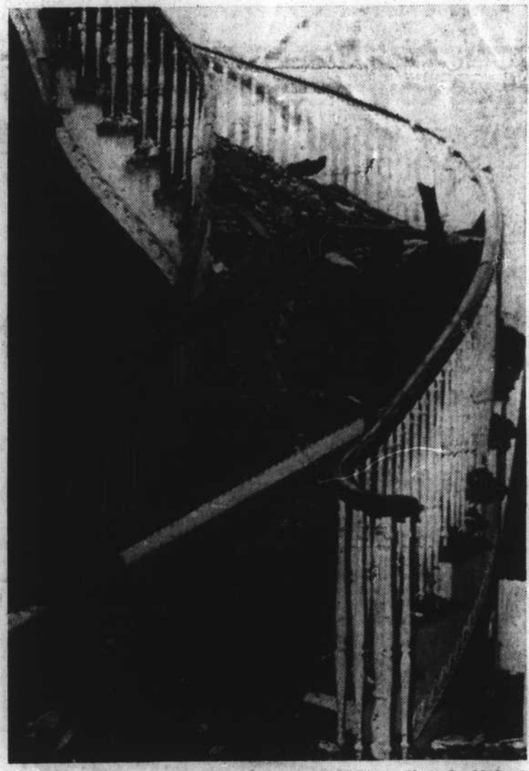
The inside of the house is a shambles. Charred wood and debris litter the staircase. Water damage was extensive. (More pictures page 8 this section.)
