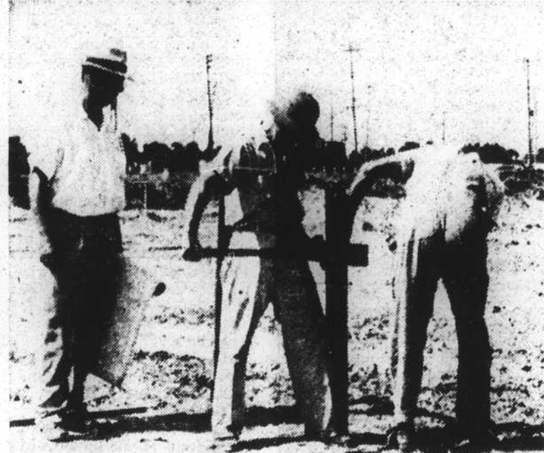
Superintendent J. W. Wheelon, Asheville, supervises preliminary work on the construction of the new National Guard armory, Morehead City. The building's outline is being surveyed and other work done prior to actual construction. Reports that a wing, headquarters for the recently-retained Army Reserve, will be added to the building, are still unofficial. Mr. Wheelon is at the left.
