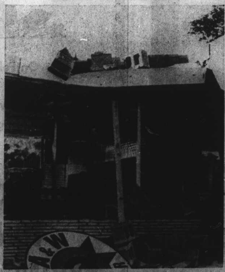
Clinder blocks and mortar litter the front of a drive-in west of Morehead City after high winds Wednesday night toppled a portion of the building. Plate glass windows were shattered under the impact. The drive-in is located on highway 70.
