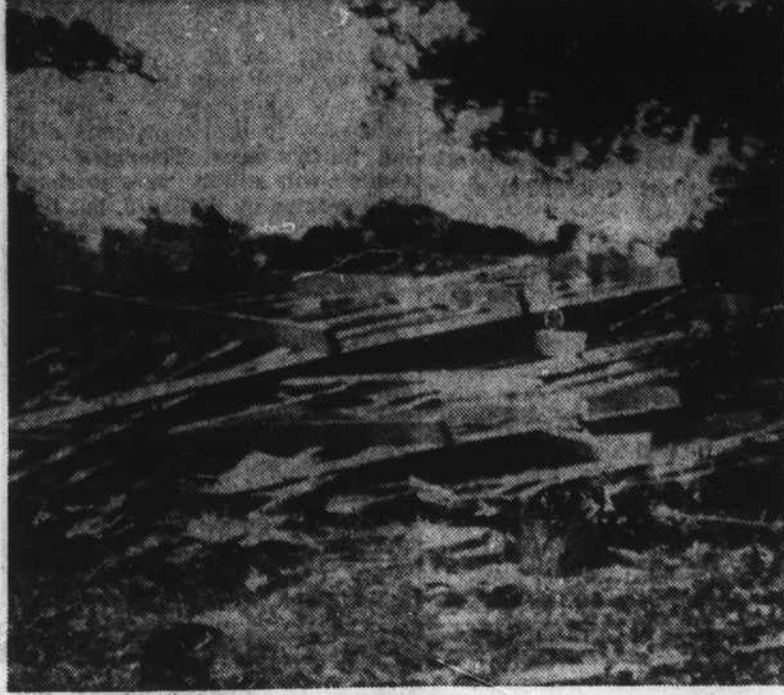
This pile of debris is all that remains of a shell shop which formerly stood in the yard at the L. T. Chesson home. Parts of the building were scattered on the highway and parts of it sailed into the woods across the highway.
