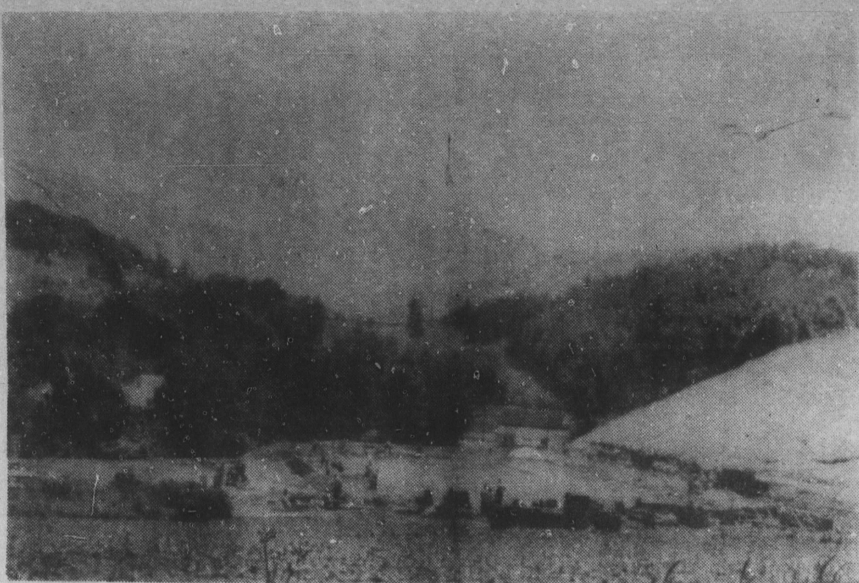
A broad view of the market building under construction in West Burnsville. Outline of the foundation blocks attests to the size.
