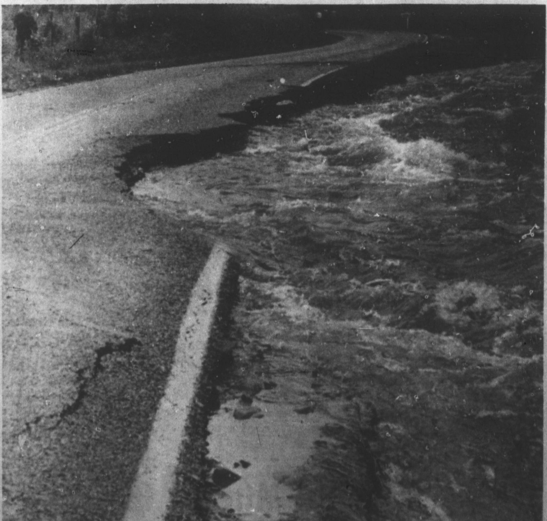
Repairing County Roads Will Be A Costly Undertaking
