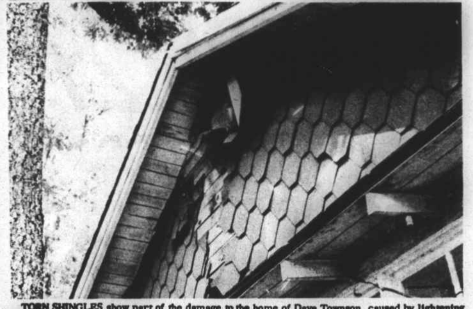
TORN SHINGLES show part of the damage to the home of Dave Townson, caused by lightning Monday morning, August 13th.
