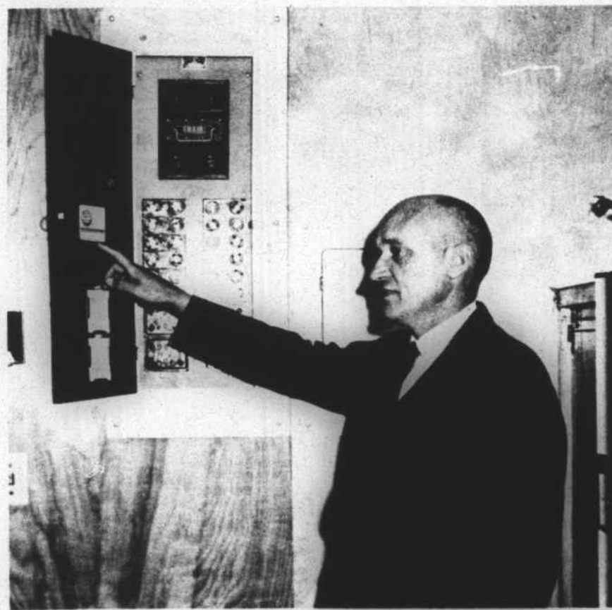
Mr. Day Points With Pride To The ADEQUATE WIRING CERTIFICATE Awarded His New Gold Medallion Home
