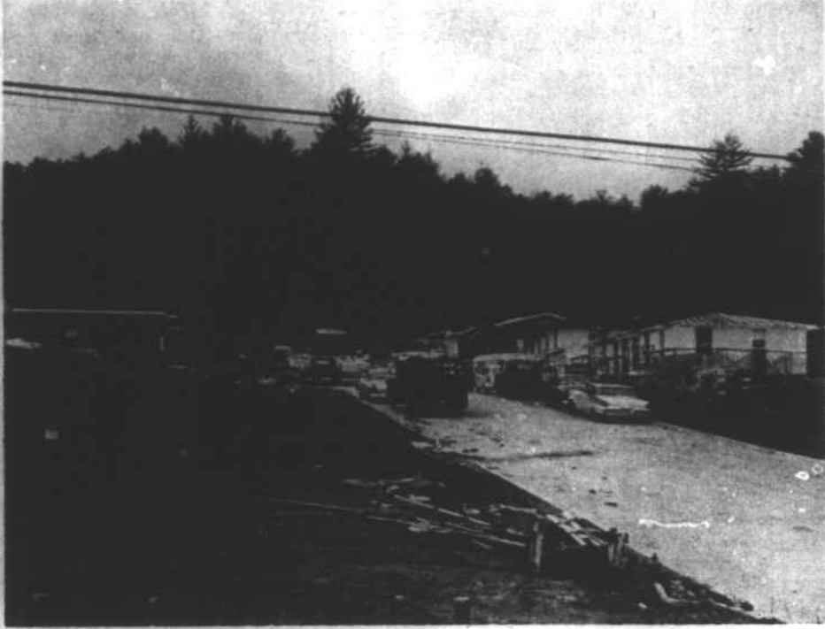
PUBLIC HOUSING PROJECT 55% COMPLETE Several of the 36 units now under construction on Hiwassee Street in Murphy, are shown in their various stages of completion.
