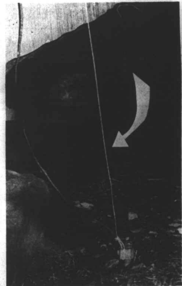
CLOTHESLINE WIRE connected to the ground wire outside the C. S. Thompson home also serves no useful purpose. The trio received only $2.00 for this installation, cutting their price from the original $217.00.
