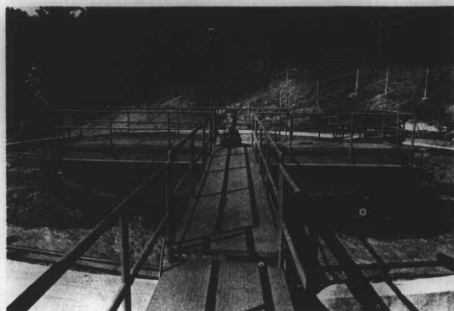
Settling basin and aerator tank which can process 500,000 gallons of sewage per day.
