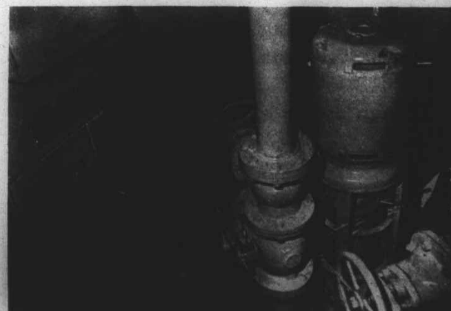
Inside of one of four new pumping stations. Eight feet in diameter and 24 feet deep.
