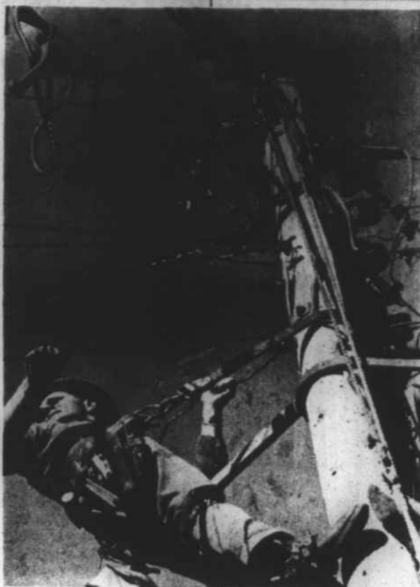
James Teems, a Nantahala Power and Light Company lineman is shown at work during the recent project to increase voltage on lines serving the Rhodo, Junaluska and Pisgah areas of Cherokee County. (NP&L Photo)
