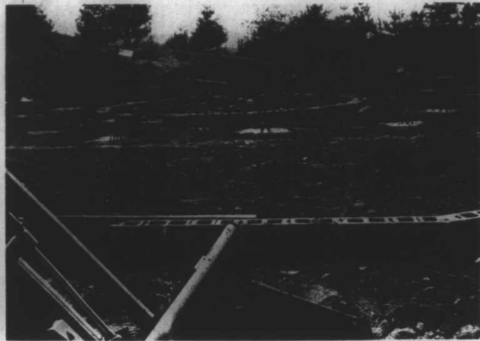
The circular shape of the additional classrooms being added to Murphy High School now under construction is beginning to become evident. The building, which will house the Junior
