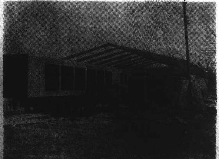
This is a pictorial progress report on the new gymnasium and vocational workshop that is being built at Adkin High School. It will not be finished in time for use during the current school year but it will be ready by next fall for the 1953-54 school year.
