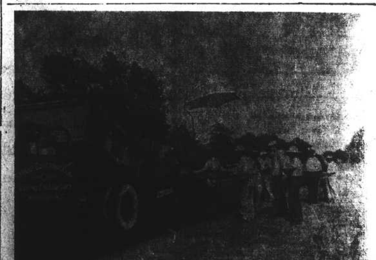
Pictured here men and equipment of the Barrus Construction Company are at work re-surfacing the Kingston-Trenton highway. This latest improvement extends from Leslie White's Store to the Trenton city limits. Other surfacing work to be done in the near future in Jones County includes the connecting road from NC 41 to NC 12 which passes Mark Smith's farm, 2.9 miles of the Black Swamp Road
