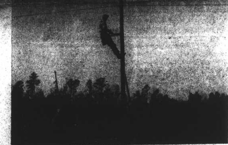
Workers pictured here are rapidly extending lines of the Carolina Telephone & Telegraph Company into the Southeastern corner of Lenoir County out the Trenton highway. This newest telephone
