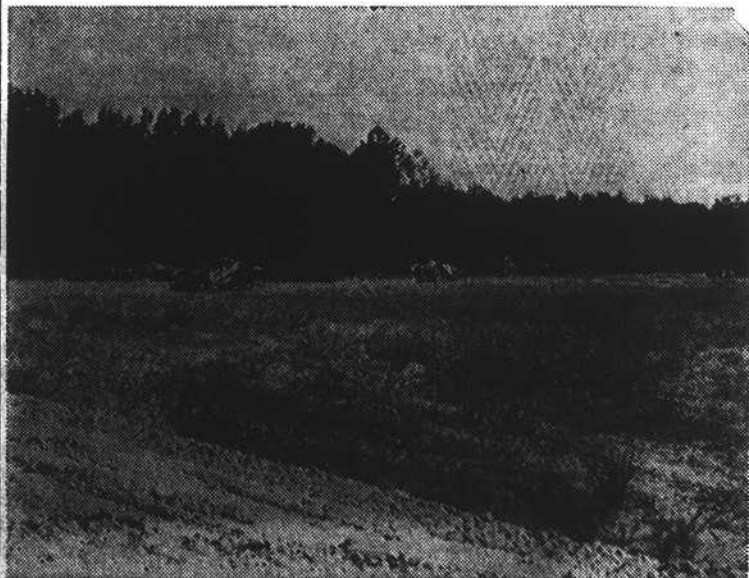
This is where the dikes are being built to form the 25-acre that will process about one-fourth of Kinston's raw sewage. When completed this dike will rise eight feet above the record flood levels ever reached by Neuse River.
