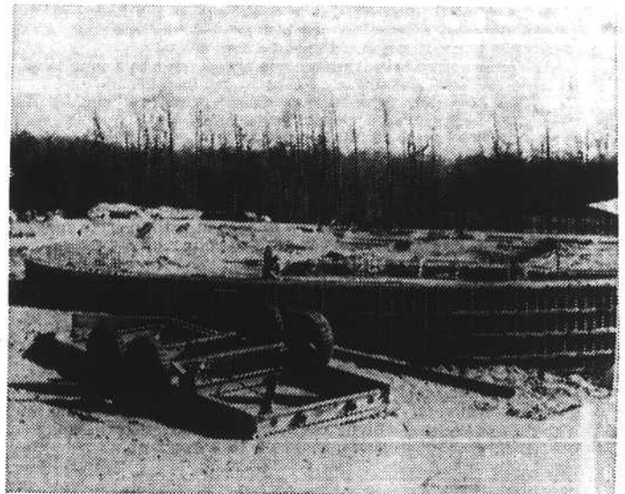
This circular chamber with reinforced concrete walls is the second basic part of the Kinston sewage treatment plant that should be finished by mid-1969. After treatment in this huge area the sewage, less some undissolved solids, will then flow into the original experimental 25-acre lagoon that the city built several years ago when a complete system of lagoons was under consideration for Kinston. From the 25-acre lagoon the finally treated liquids will then be returned to Neuse River through a canal system, which will parallel the right of way of the Atlantic and East Carolina Railroad.
