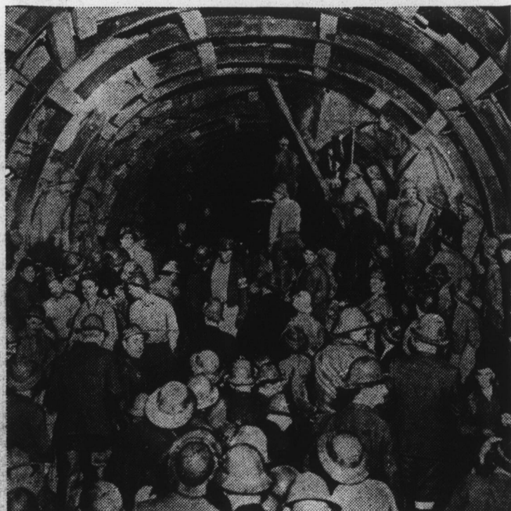
Completing a five-year job, hard-rock men holed through in the San Jacinto tunnel recently. Within a few months 1,000,000,000 gallons of the Colorado river will rush through this 13-mile bore daily in its haste to quench the thirst of Los Angeles and 12 other southern cities. It was one of the biggest tunneling jobs ever attempted.
