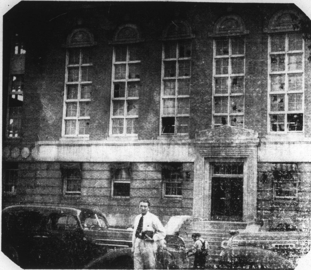
This broad view of the South side of the Person County Court House shows windows broken by flying pop bottles, rocks and gunfire. Windows have now been replaced. The jail is on top floor of the Court House. Most of the damage was done about 2 A. M. Saturday. Photo by Person County Times.
