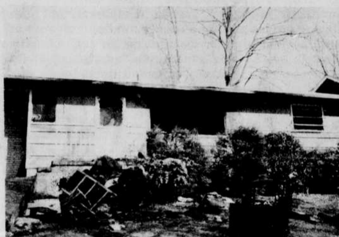
The exterior of the house was not so severely damaged as was the interior and its contents.
