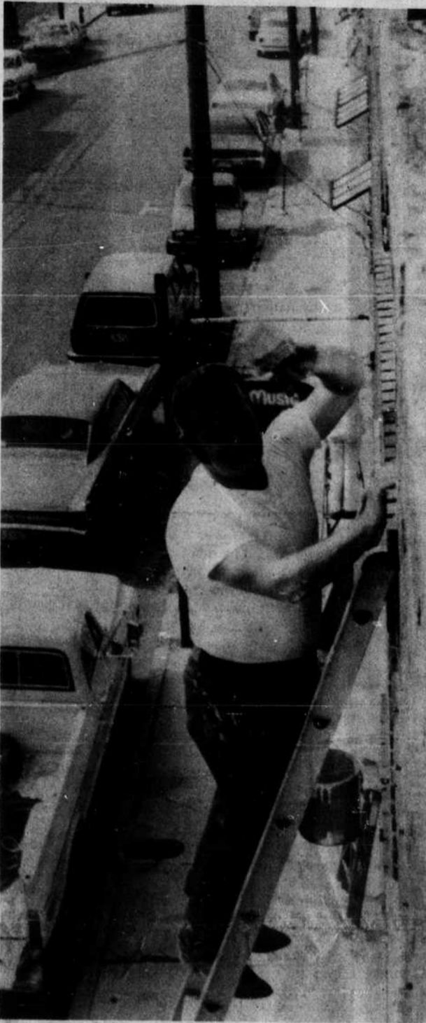
JAMES NANNEY, of Nanney's Repair Service, puts the finishing touch on an upstairs window frame at the antique shop on Cherry St. (Dan Ward)
