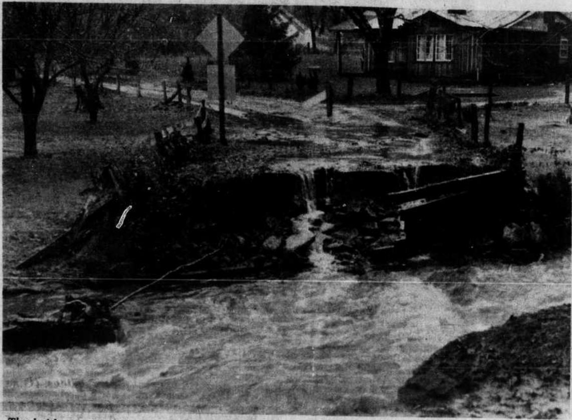
The bridge at Flat Creek and Montreat Road washed away. (David Peele)
