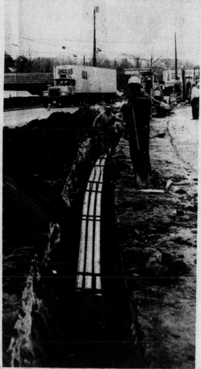
Workers lay conduit through which telephone circuits will be pulled next year. (Dan Ward)
