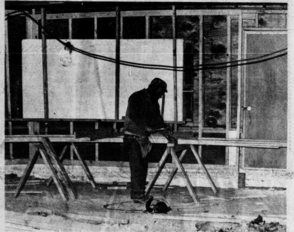
A carpenter does some work on renovating the lower floor of the Black Mountain Clubhouse for senior citizen use. The lower floor, when completed, will be known as the Lakeview Multiservice Center for the Aged. (Dan Ward)
