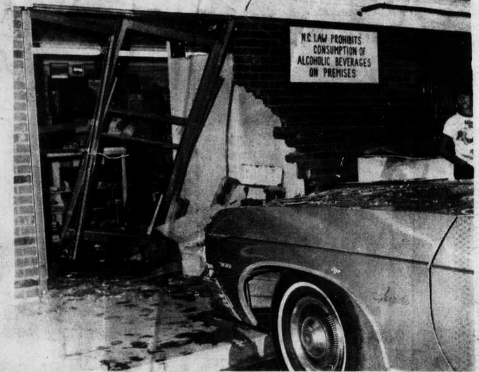
Burton's Package Store experienced extra ventilation last week when the car driven by a Black Mountain woman crashed through the door. (see related story) (Gary Sorrels)
