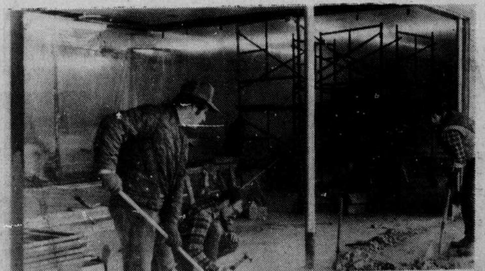
Renovations are underway at the new home of the Black Mountain News.
