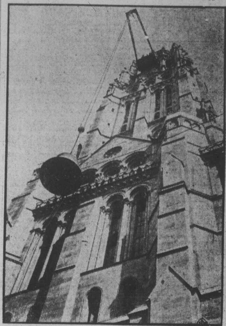
The 22-ton Bourbon bell, which completes the largest carillon in the world, being hoisted up the front of the new Riverside Church, on Riverside Drive and 121st street, New York City.
