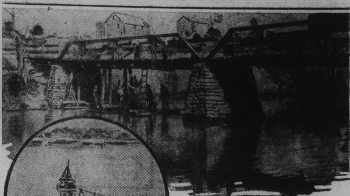
With work on the Tennessee Valley project, keystone of the Public Works program, being pushed forward, workers believe in strengthening their bridges before they cross them. Above, a bridge of ancient vintage, near Knoxville, Tenn., is undergoing rigid reconstruction to enable it to safely bear the heavy trucks going to and from Wheeler Dam site. At left, dredging barges are shown at work on the site of the dam that will be more than a mile long and will form a lake of more than 100 square miles.
