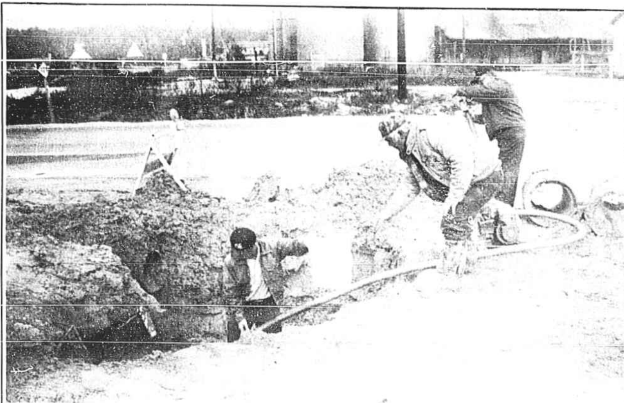
SHALLOTTE TOWN EMPLOYEES, from left, Danny Roden, Isaac Ward and Roland Varnam use a motorized pump and buckets to remove water from around a
