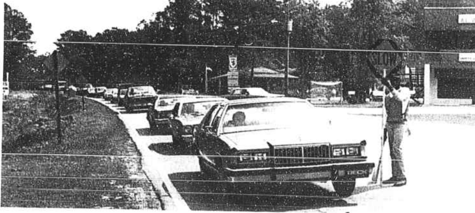
FLAGMAN DEMPSEY FLOWERS of Chadbourn stops traffic last week on U.S. 17 South in Shallotte, as road crews from Dickerson Carolina Inc. of Castle Hayne begin resurfacing the highway from the town
